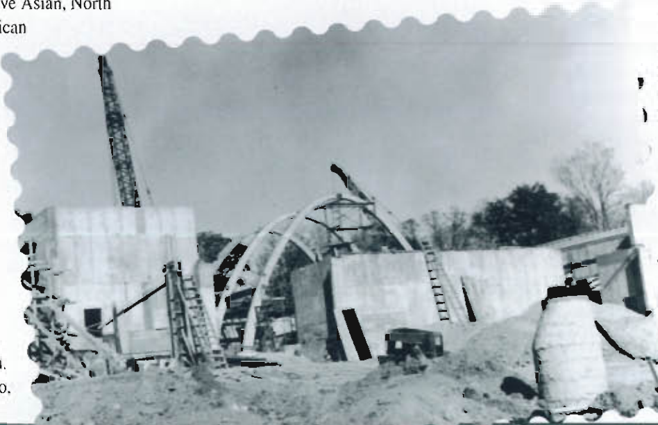
The new Zoo started to take shape in the late 1950s, when construction began on the Primate Building, Monkey Island, Feline House, Pachyderm Mall and Grizzly Bear Den. The Feline House under construction is pictured here.
