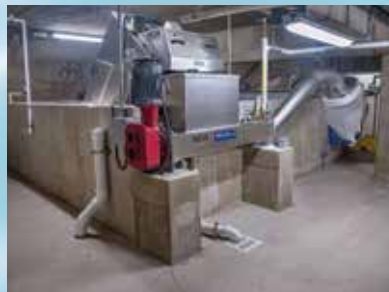
A press squeezes the water out of the waste to allow for the removal of a lighter product.
