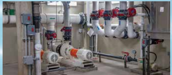
The jet pumps are set on a timer to turn on and scour the bottom of the outdoor exhibit to remove debris.
