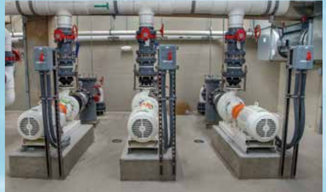
▲ The three main pumps push the water at a rate of approximately 2,640 gallons a minute.
