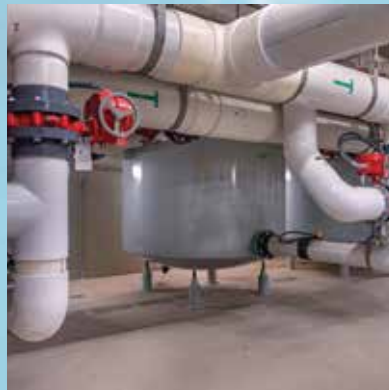
▲ The system includes five sand filters that remove fine solids from the recirculating water.
