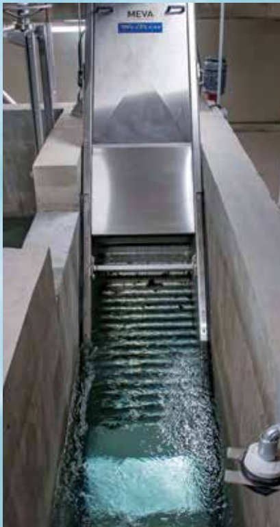
Monoscreen filters remove larger solids from the water returning to the pump from the outdoor exhibit.
