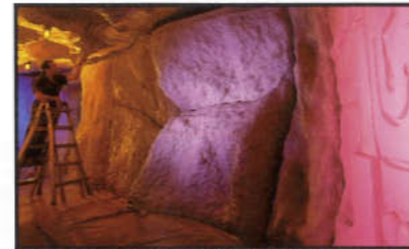
Building the butterfly exhibit's "ruins"; Richard Nebel of ACME Corp. finishes painting a Belizean "cave" with a Maya glyph on the wall.
