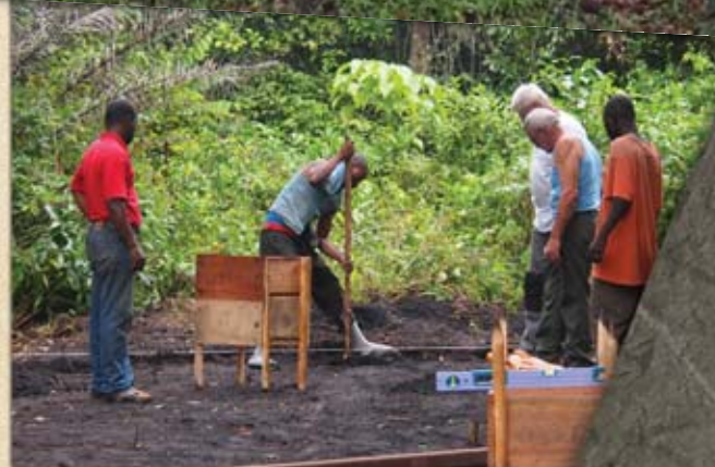
With supervision from construction experts, guards begin the foundation for an elevated house at Etate.
