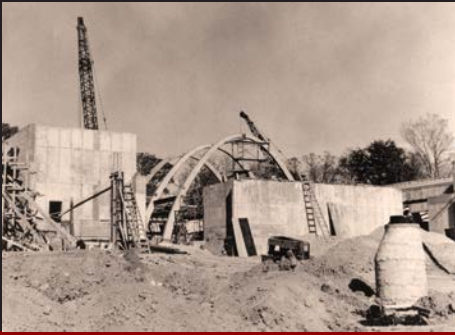
Construction of the Zoo's feline house began in the 1950s. Photo courtesy of Milwaukee County Zoo Archives
