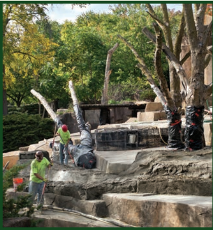
Workers from Cost of Wisconsin, Inc., renovate the Black Bear Exhibit. Photo by Richard Brodzeller
