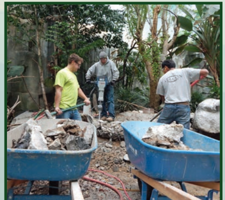
Workers from Allcon Construction LLC remove granite to allow machinery to reach parts of the Free Flight Area. Photo by Zak Mazur
