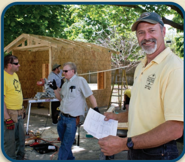
Andy Hemken (right) examines blueprints for the new beehive building during its construction in May.
